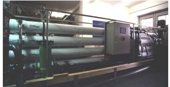
RO240 system, Iran, Fresh Water Application
